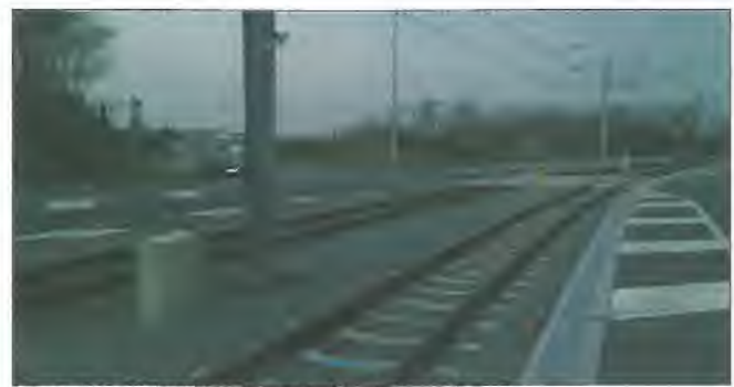
Fig. 7: The APT-WORM installed on ballasted track
