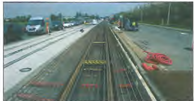
Fig. 8: The APT-WORM installed in a newly-built track
